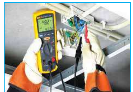
Insulation Resistance Test
